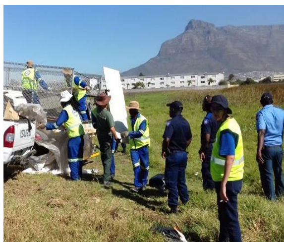
Figure 56: Illegal structures removed from a reserve.
